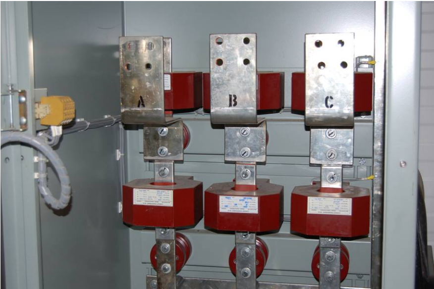
Photo 5.4: inside of power factor capacitor cell 4-U-2.
