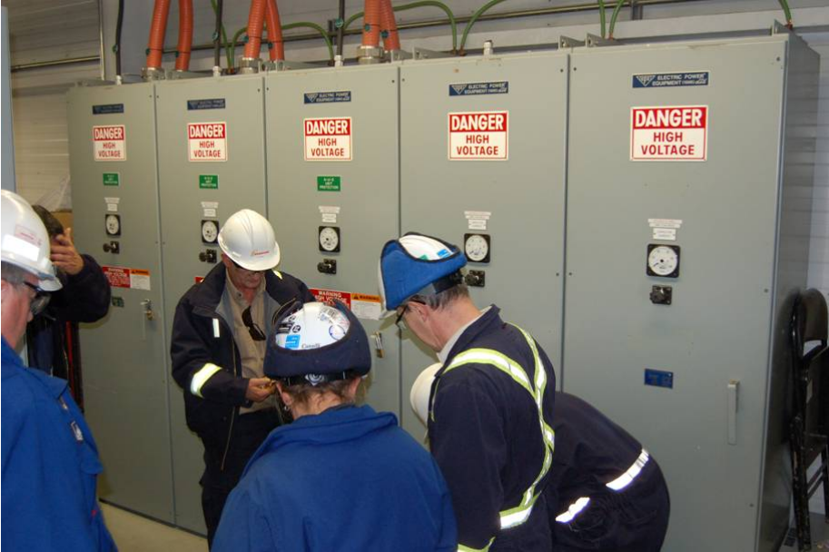
Photo 5.3: Power factor capacitor cells.
