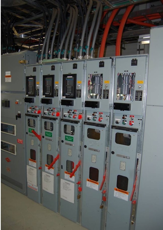
Photo 5.1: Unit starters located in 4-ESB-1 building.
